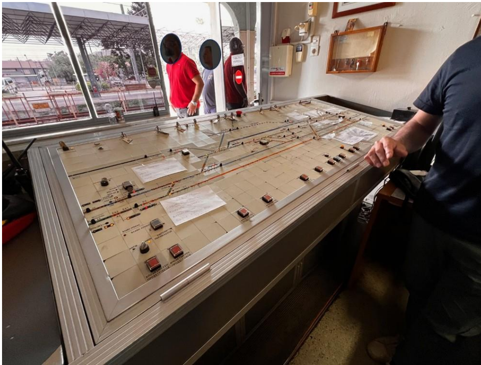
Figure 37. The control panel at Larissa Station
